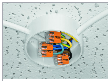
Lighting distribution in ceiling canopy
